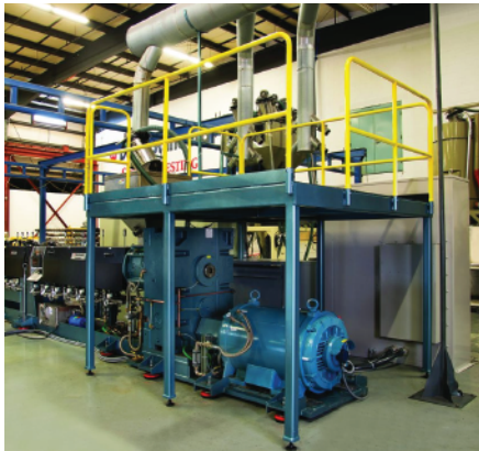
EQUIPMENT SUPPORT STRUCTURE
